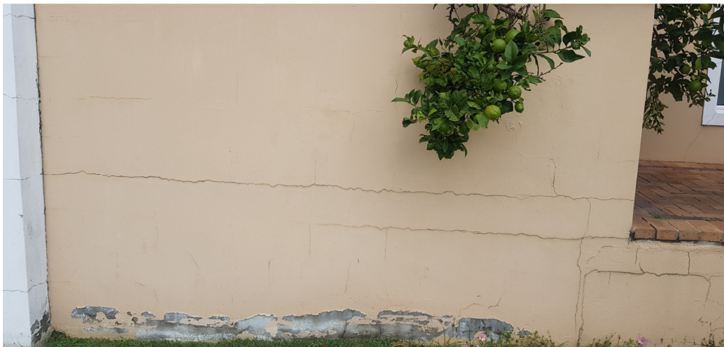
Photograph 10 - Typical external wall cracks
