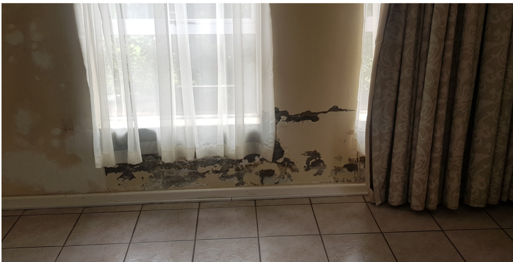
Photograph 1 – Northern Elevation Lounge area internal wall damage
