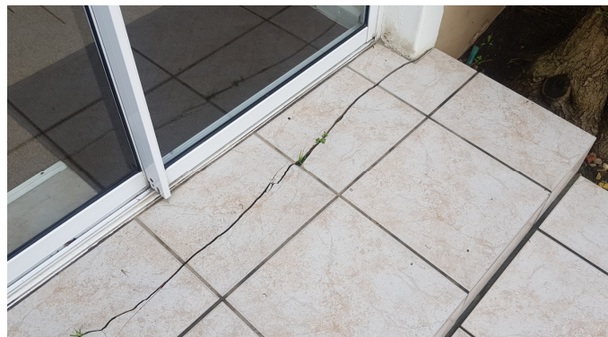
Photograph 12 - Settlement at steps leading from bedroom
