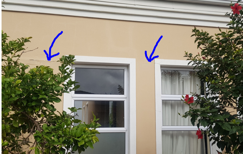
Photograph 2 - External view of Northern Lounge wall, note damage at window lintol level
