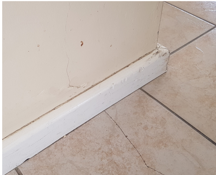
Photograph 6 – Example of cracks observed
