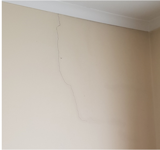
Photograph 5 - Example of typical cracks observed (1-2mm)
