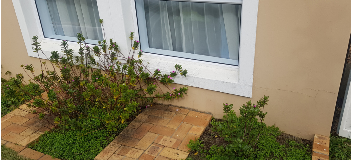
Photograph 4 - No Weepholes to external wall
