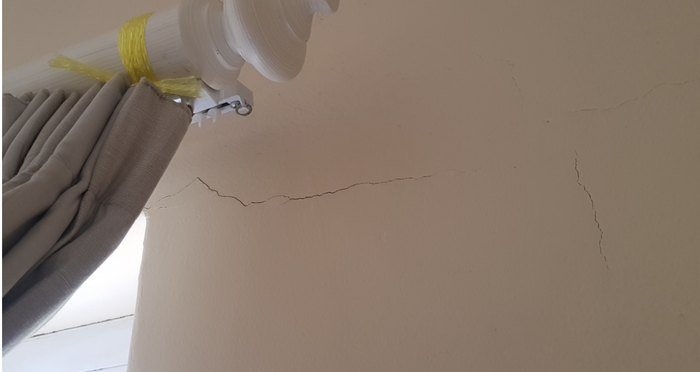
Photograph 7 - Example of cracks observed
