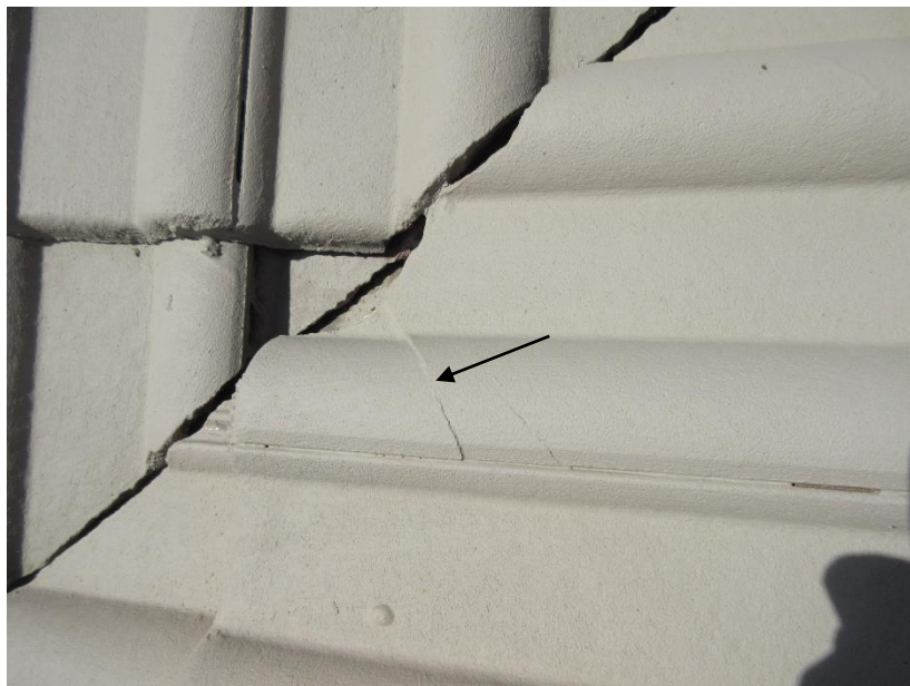
A cracked tile that has simply been painted over.
