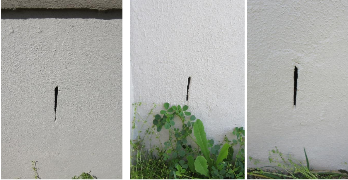
Three separate weep holes in the same wall. Note how they vary in width and height and the middle one is not even plumb.
