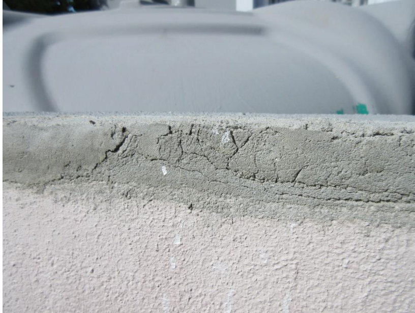
Further evidence of very poor quality and inferior plaster work.
