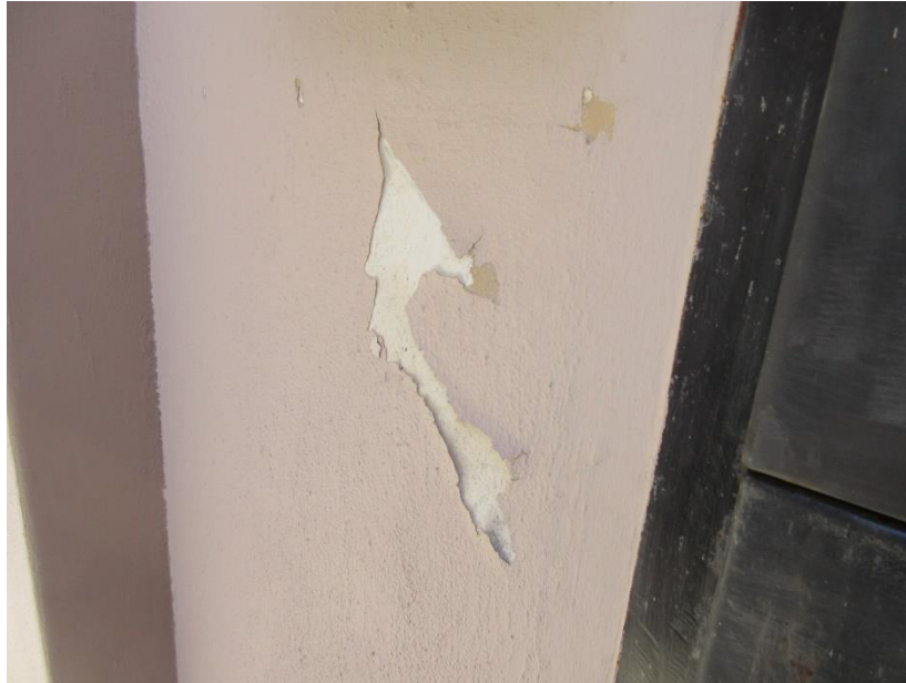
Evidence of paint peeling off at the braai area.
