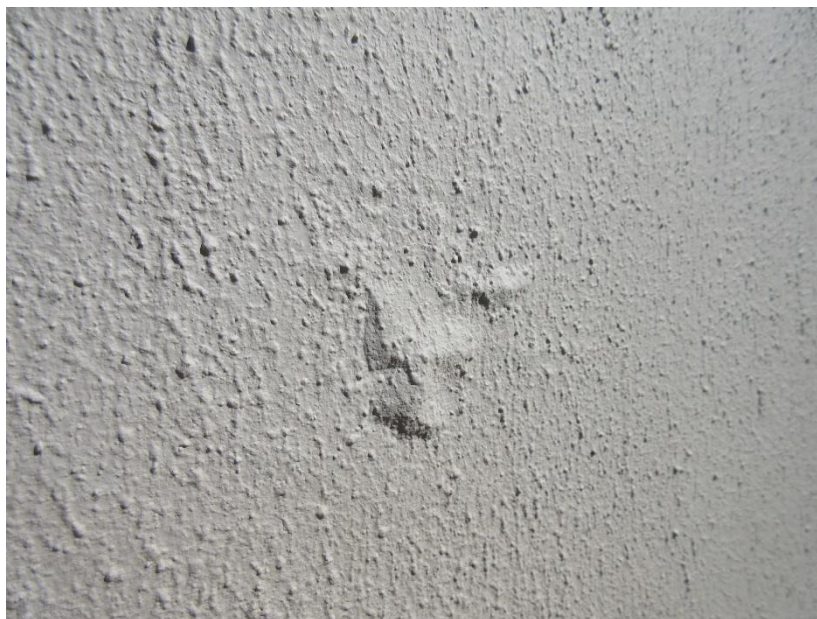
Evidence of paint bubbling and flaking on the wall surface due to high moisture content in the wall.
