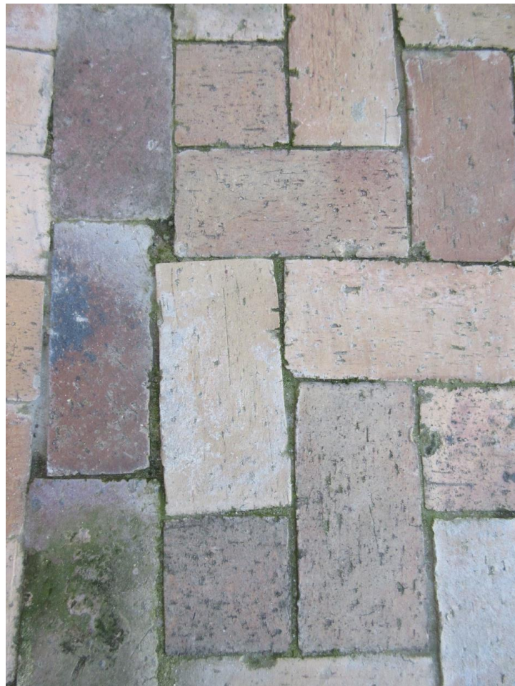
Evidence of very poor quality brickpaving with cut bricks and wide gaps between bricks.
