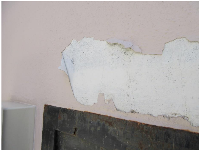
Where this paint has peeled off, there is a powdery surface on the wall.
