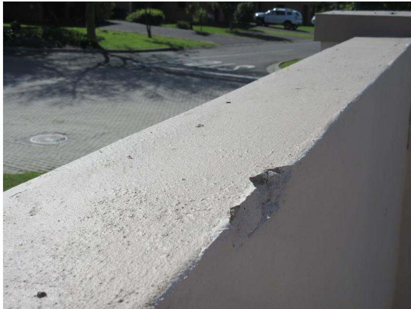
This damaged wall has simply been painted over.
