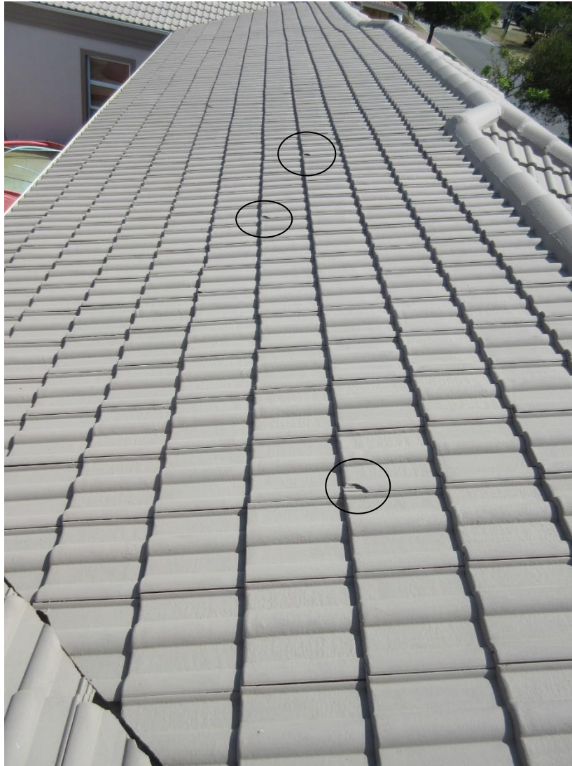
More cracked and broken tiles that have simply been painted over.
