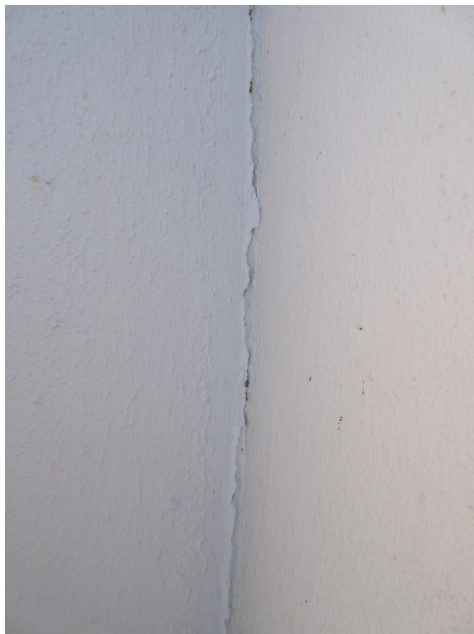
Evidence of a crack reoccurring between two wall surfaces.
